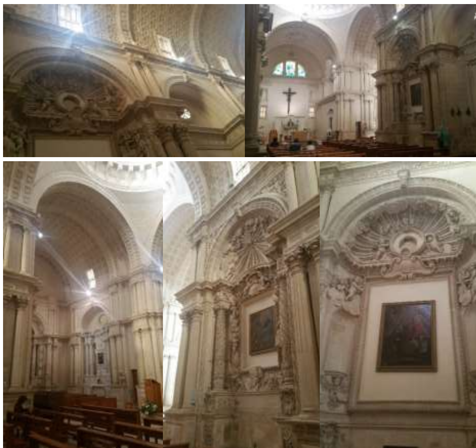
Fig. 2. Part of photographic survey of the Old Parish Church of Saint Mary, Birkirkara, undertaken by Jovan Stefanovski (© Jovan Stefanovski Archive)
